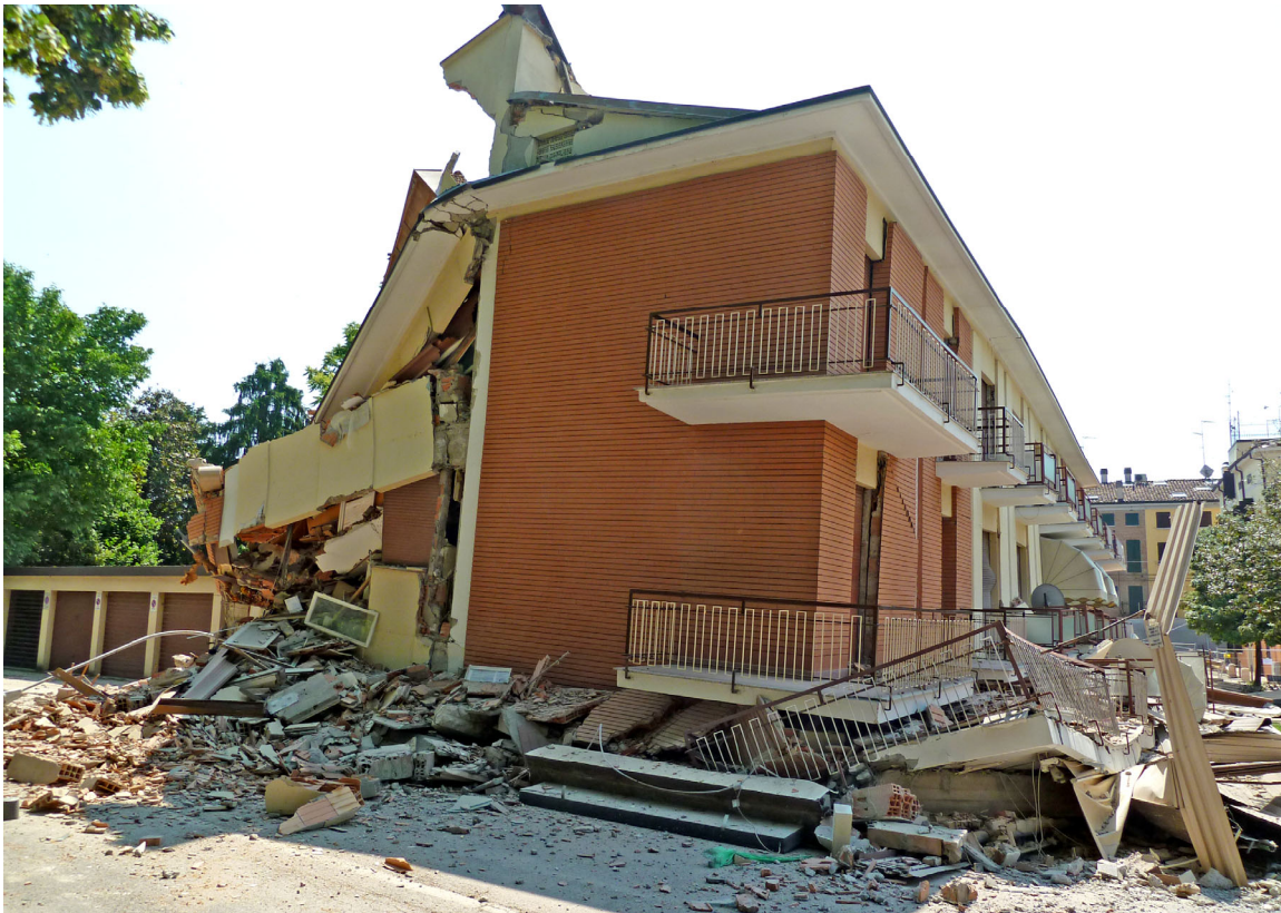
Fig. 14 - Cavezzo (Is 7 MCS). Total collapse of the pilotis of a r.c. building in the old-centre (photo of May 29). This building experienced level 2 damage because the May 20 mainshock, and was not inhabited when it crushed on May 29.
