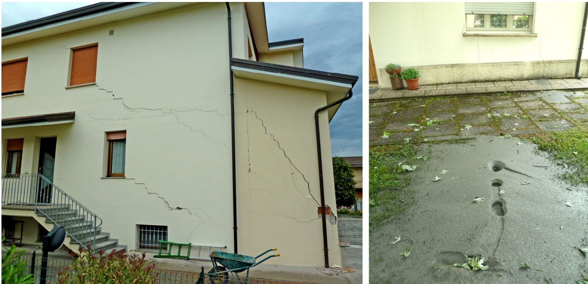
Fig. 17 - San Carlo: left, differential settlement of a mixed r.c. and masonry building, due to huge liquefaction phenomena below part of the foundation. Right, sand ejected from a water-manhole (photo of May, 20).
