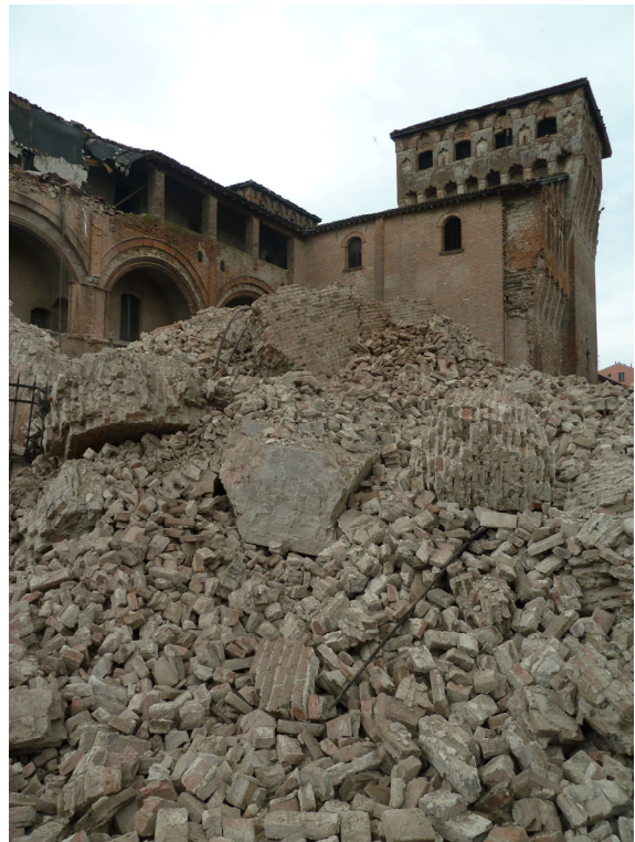
Fig. 7 - Partial collapse of the Estense castle (15th century) in Finale Emilia ( I_s 6-7 MCS) in the morning of May 20.
