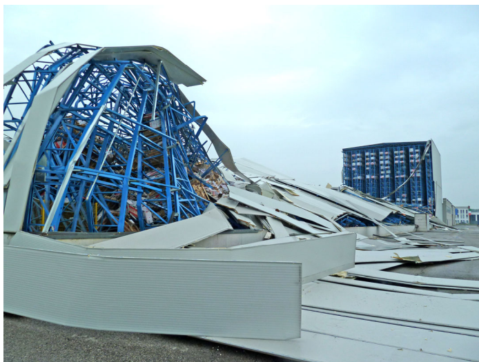
Fig. 9 - Collapse of the Sant'Agostino's ceramics warehouse.
