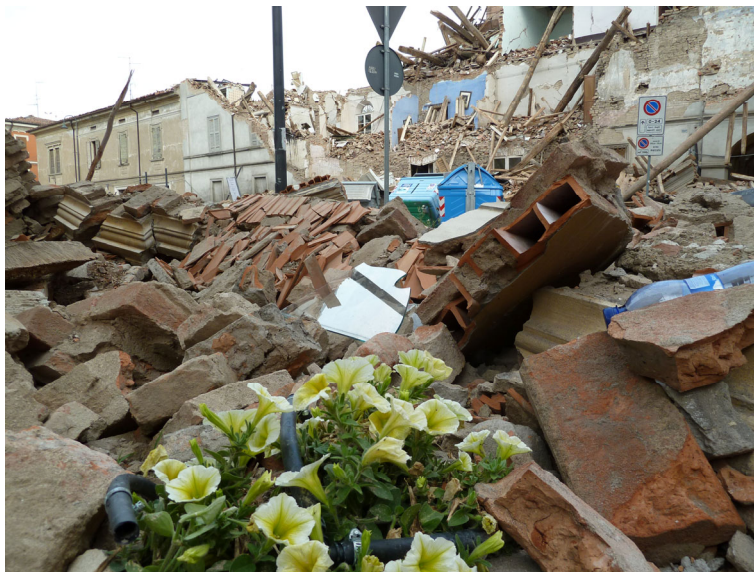
Fig. 12 - Concordia sulla Secchia (Is 7 MCS). Collapse of inhabited, old unreinforced brick-masonry buildings inside the old-centre (photo of June 6).
