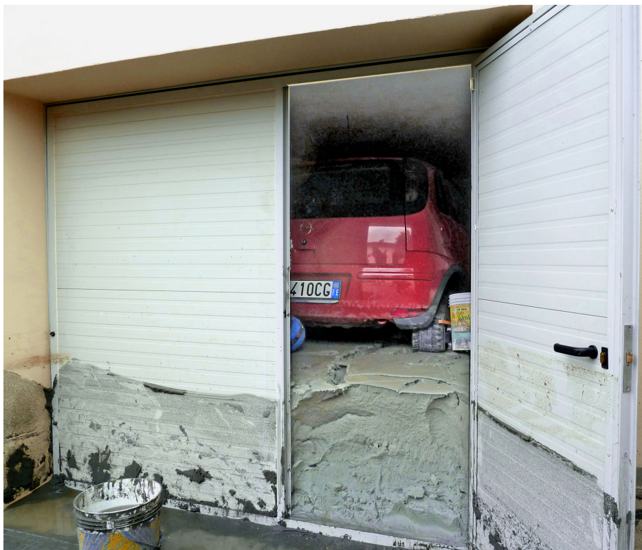
Fig. 20 - San Carlo. Sand ejection inside a car-box. Remarkably, that the car has been by raised by ~80 cm up to the ceiling of the box due to the powerful push of the liquefied sand below during the night of May 20. This side of the house (see Fig. 17, left) has been severely damaged by differential settlement.
