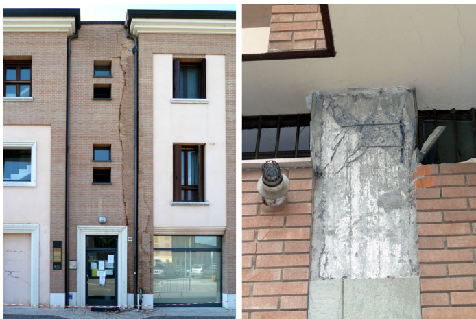
Fig. 10 - Left, Cavezzo (Is 6 MCS), May 22: level 3-4 damage along the joint of a r.c. building inside the old-center; this building collapsed entirely because of the mainshock of May 29. Right, Mirandola (Is 7 MCS), May 21: crushing of a pillar of a r.c. building in the old-centre.
