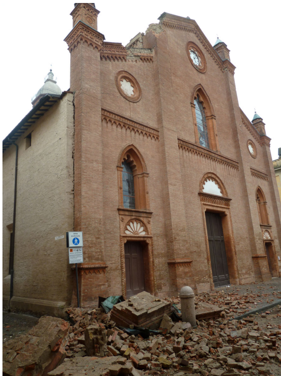
Fig. 6 - View of the Mirandola Cathedral (15th century) in the morning of May 20. At that time, only few architectural elements at the top of the façade were fallen down, beside the incipient façade detachment. Inside, not visible, also part of the roof has fallen down. The church was damaged again, more seriously, by the May 29 mainshock.
