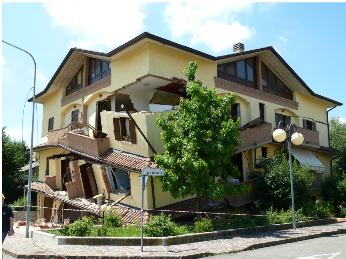
Fig. 15 - The impressive collapse of the brick-masonry pilotis of a new building in the outskirts of Rovereto (Is=Imax 7-8 MCS).
