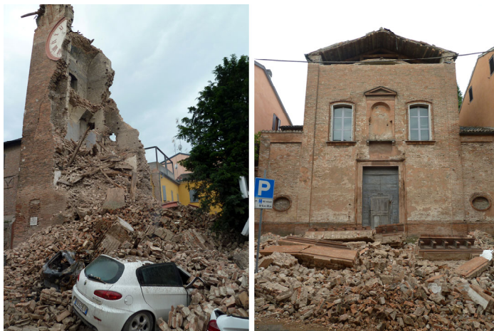
Fig. 8 - Finale Emilia (Is 6-7 MCS): collapse of the Medieval clock-tower, and of the Cathedral tympanum in the May 20 morning. The tower collapsed definitely during the seismic sequence.
