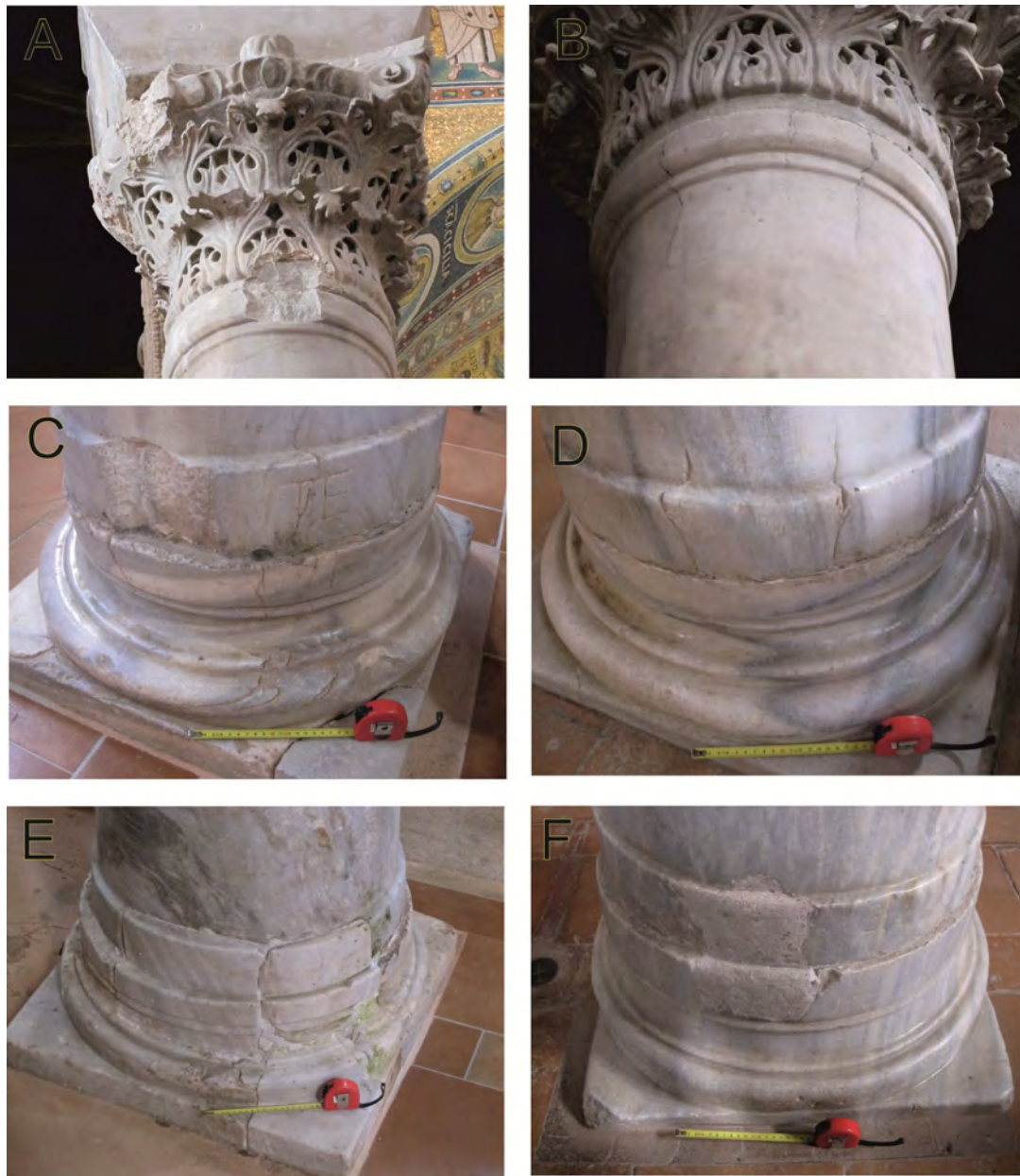
Fig. 6 - Fractured capitals, pillars, and plinths. Fracture planes are vertical, parallel with the axis of the columns, indicating the dominance of vertical shaking. A. Fully developed adjacent fracture both in the pillar and the capital. Pillar F, capital. ADB photo #0080. B. Two, conjugate joints enclose a slice of marble. If this fracture had developed further, a thin flake of stone would have been removed from the capital (see the similar feature demonstrated by Ambraseys & Psycharis, 2012, their fig. 8(b)). Pillar N, capital. ADB photo #0082. C. Broken-off corner of a pillar. An adjacent fracture marks the place where a second break-off might initiate. Pillar A, plinth. ADB photo #0076. D. Initial fracture, bordered by conjugate joints. Pillar O, plinth. ADB photo #0087. E. Broken-off splinter replaced by marble. Note the misfit of the column and the plinth: the column is narrower. Pillar I, plinth. ADB photo #0081. F. Missing splinter, repaired by concrete. Note the misfit of the column and the plinth: the column is wider. Pillar N, plinth. ADB photo #0086.
